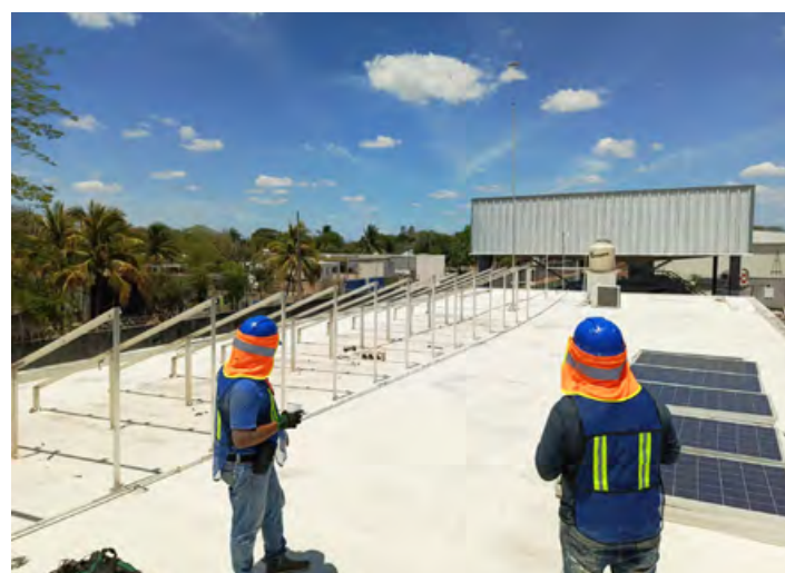
Solar power generation systems, Mérida Airport
